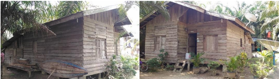
Figure 3 Condition of the Bonai Tribe's House
